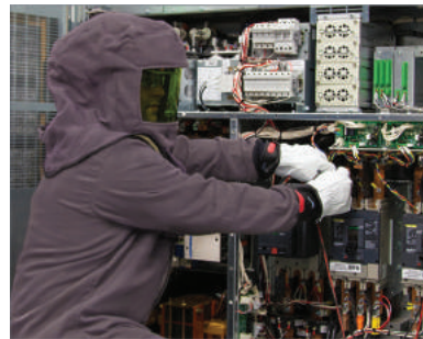
Service: • AMC • Mission Critical Facilities Management Services
